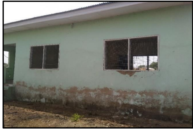
Picture 7.14: An abandoned house at the Dokokyina resettlement community showing a damp, peeling and cracked wall (Source: E. Agyepong, 14 December 2018)
