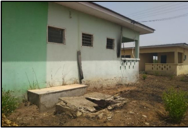
Picture 7.15: An abandoned house at the Dokokyina resettlement community showing a collapsed manhole and exposed electrical wires (Source: E. Agyepong, 3 March 2019)
