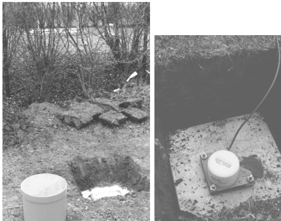
Figure A.5: Hollow for a platform tiltmeter at PLT8 OE , with B2 OE in background behind the bushes (left), and installed instrument, AGI 701-2 (right, arranged).
