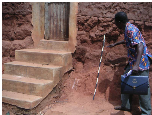
Fig. 10: Extend of erosion processes on the 'terre de barre' examined in the village of Oudeme-Peda in southern Benin (Photo: J. RÖHRIG, 2006)
