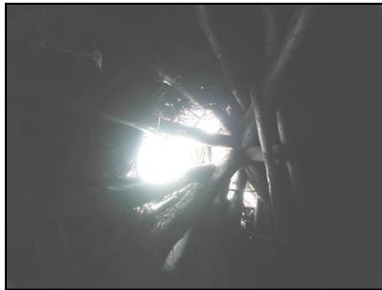
Figure 2.3 A broken grass-thatched roof
