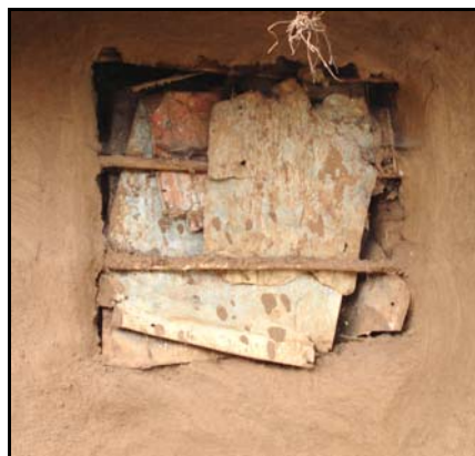
Figure 2.5 Window fixed with old pieces of metal
