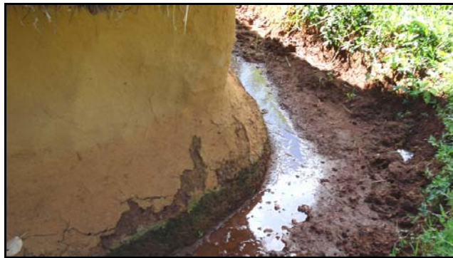
Figure 2.8 Stagnant water around a house
