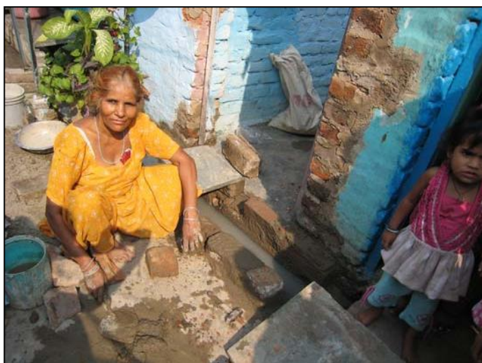
Photo 8: Building infrastructure. A woman raises the walls of the drains with bricks in order to avoid overflow. (Photo: A. Zimmer, November 02, 2008)
