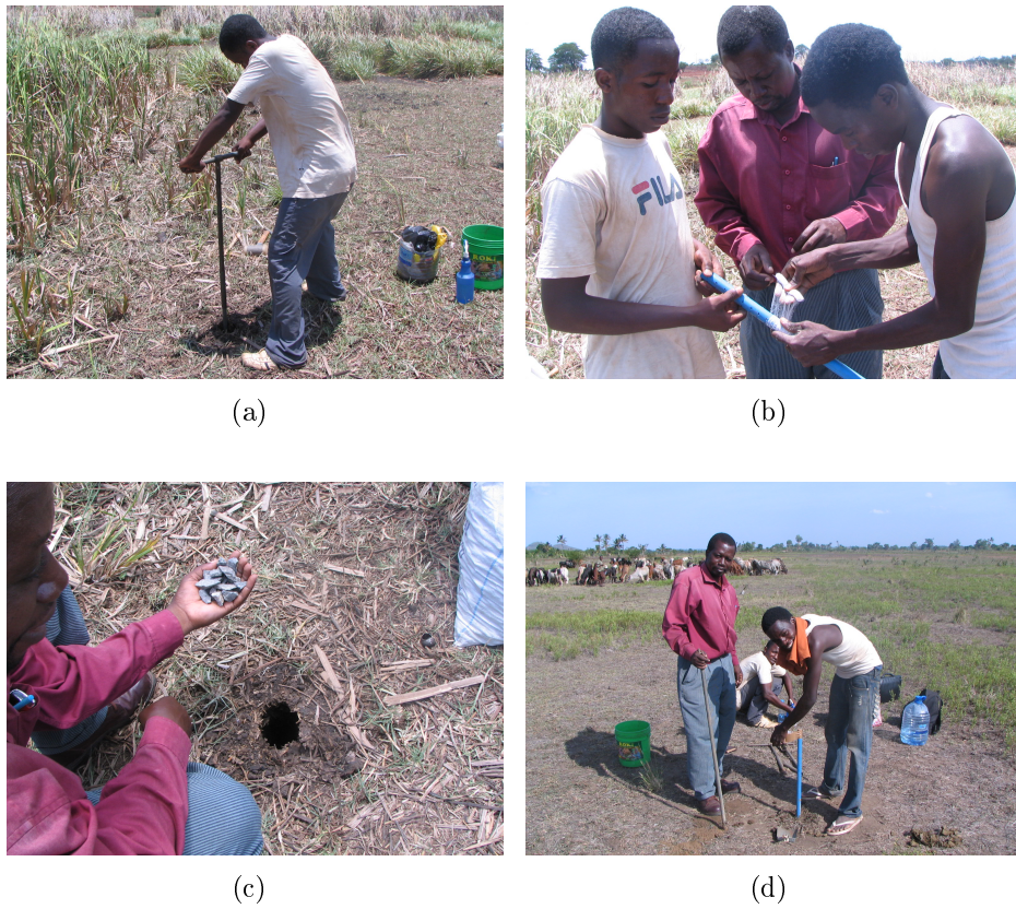
Figure B.1: Installation of piezometer: (a) Drilling of 2 m deep hole; (b) Perforation of pipe. Slots are covered with a bandage to prevent clogging; (c) Bottom of hole up to upper end of slotted portion of pipe filled up with gravel; (d) Operational piezometer.
