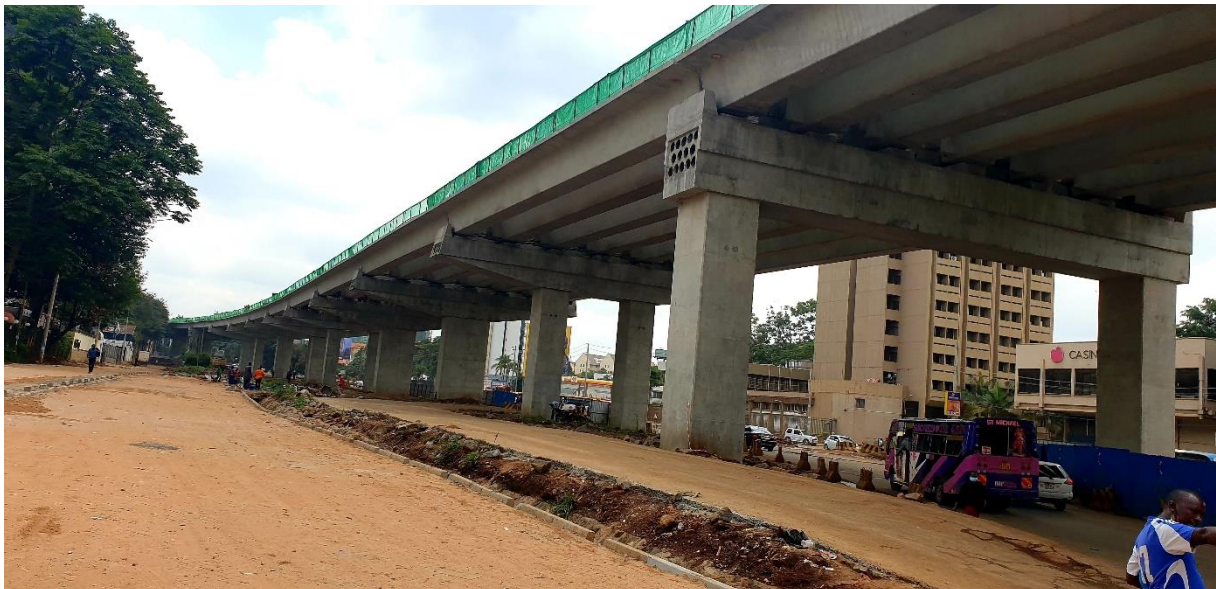
Figure 11 A section in Westlands of the Nairobi expressway under construction. Photo: A.Ogolla 2021
