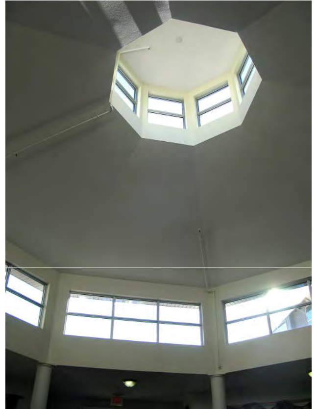
Pic. 118 a: Mountain Village, octagonal-shaped entrance ceiling Source: Courtesy of Philip MacDonald
