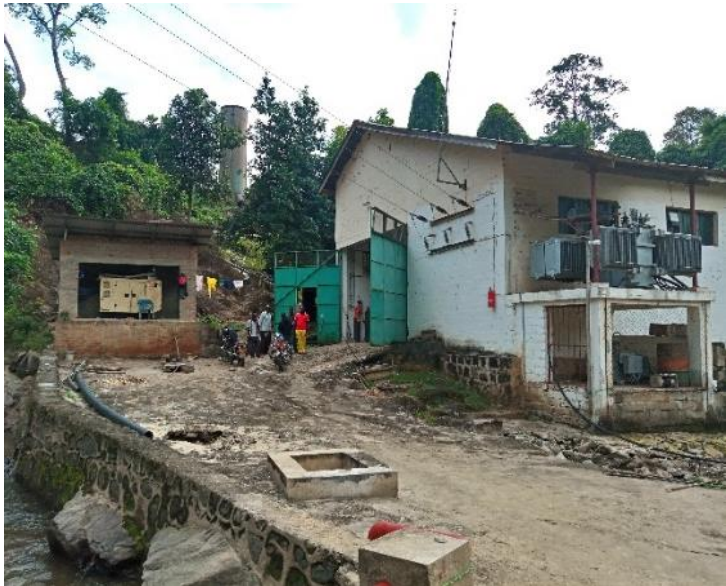
Figure 31: Electrification of the Kilombero Valley (photos: RV)
