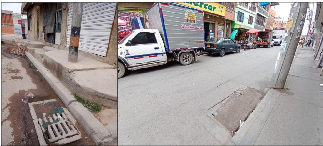
Catchbasins are covered by community members due to unpleasant odors.
