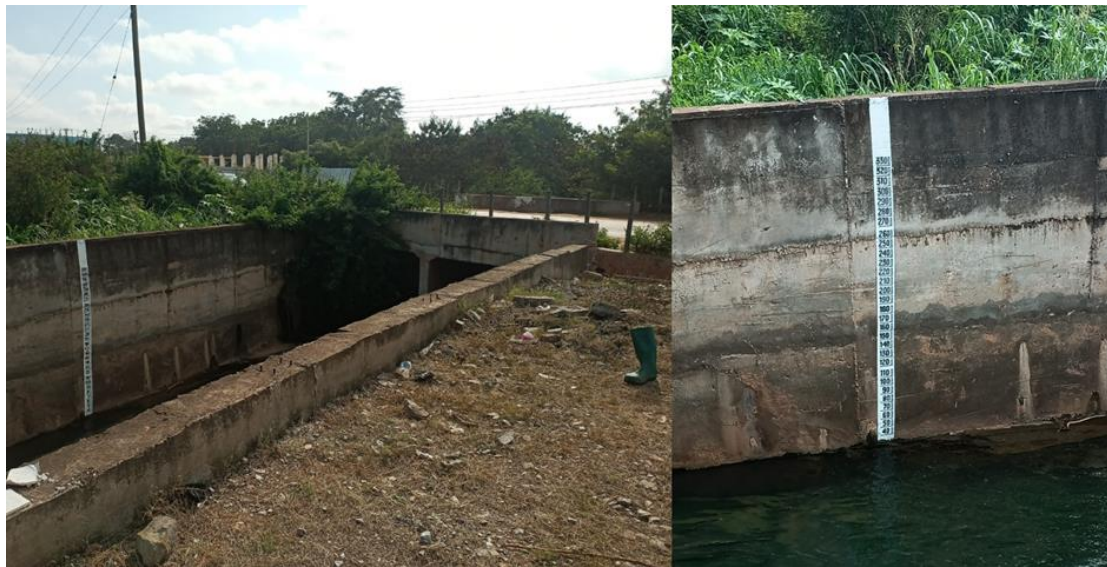
Figure 14. Scale placement for community gauge: Haatso right after installation. © WRC
