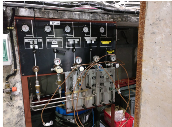
(b) Control room
