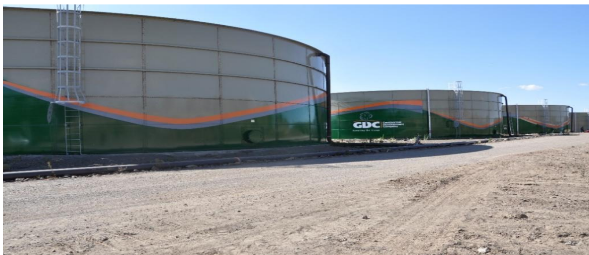
Figure 4: Menengai geothermal project water storage systems
