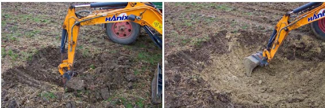
Figure 10.3 Digging and loading of the clay soil at Frankenforst research station, 9 th of February 2005: left upper layer, right lower layer
