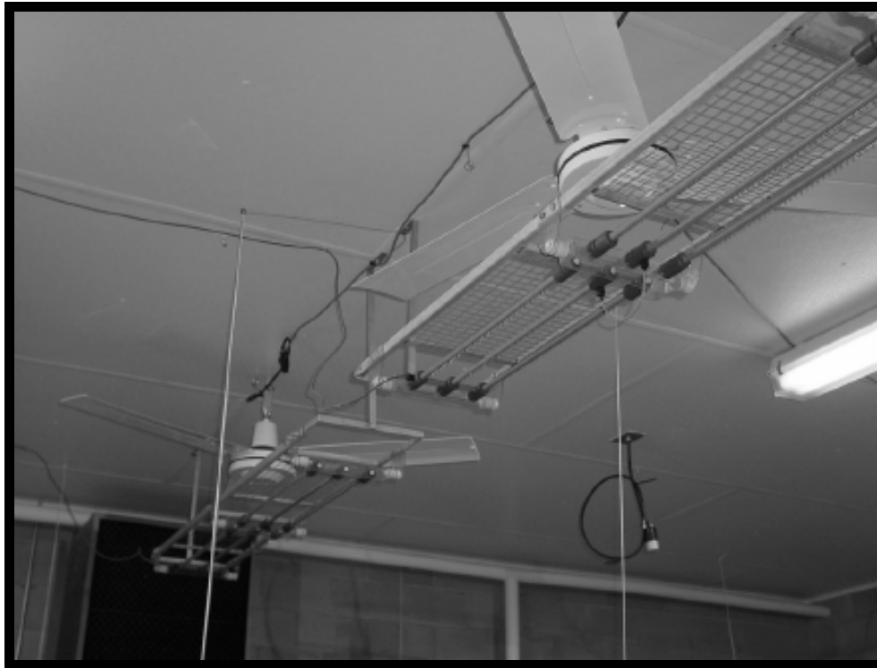
Figure 2.33: ESCS units suspended below the ceiling fans in the treatment room (Mitchell et al., 2004)
