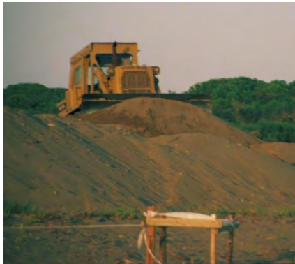
Figure 4.10 a: Construction site (Section II). Sand-mining. In the front: sea turtle nest
