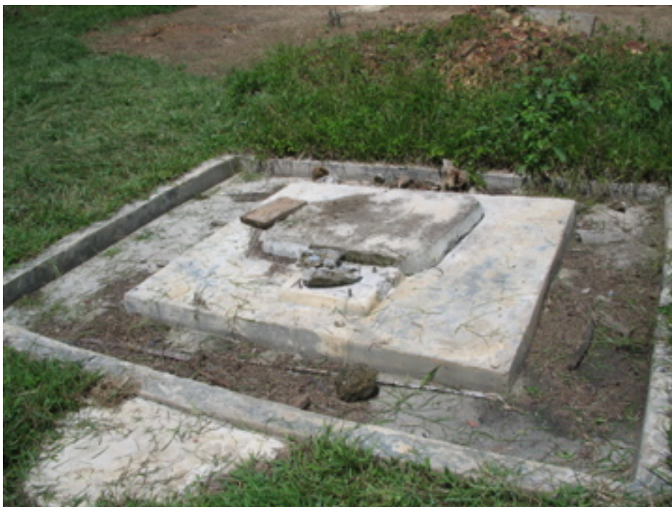
Picture 5-4: Showing one the Non-Functional Boreholes in Tebe Village
