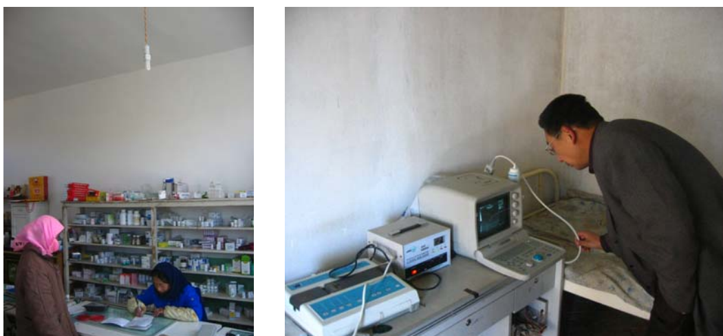
Photograph 7-6 Lighting situation at the Namcuo Township Health Center (left) and electrical medical equipments at the Saierlong Township Health Center (right)
