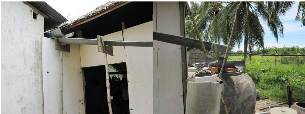
Figure 1a – Rainwater harvesting system at a rural household in the Hau Giang Province. Rainwater is collected from roof-tops by gutters (left picture) and transported to storage basins (right picture). This household indicated to use the collected rainwater for drinking (source: Author, 2011).
