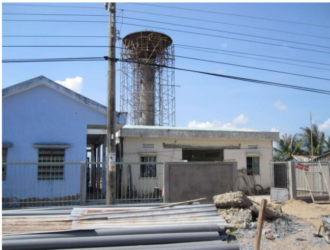
Figure 1d – Development of a water supply station in the rural areas of Soc Trang province. The image shows the construction of a water storage tower and the transportation pipes to connect households to the supply station. Behind the two houses (not visible on picture) the water treatment facility will be developed (source: Author, 2012).
