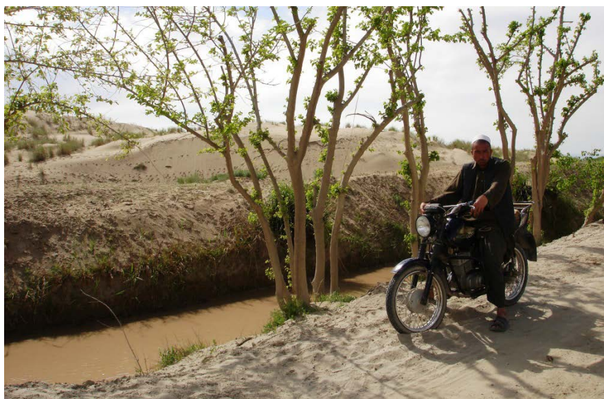
Photo P2: Canal bank erosion Qal'a-ye Zāl
