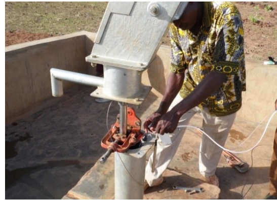
Fig. 4-4 Installation of a deep groundwater piezometer in a local pump at Gninkpière (see Fig. 4-7 for the location).
