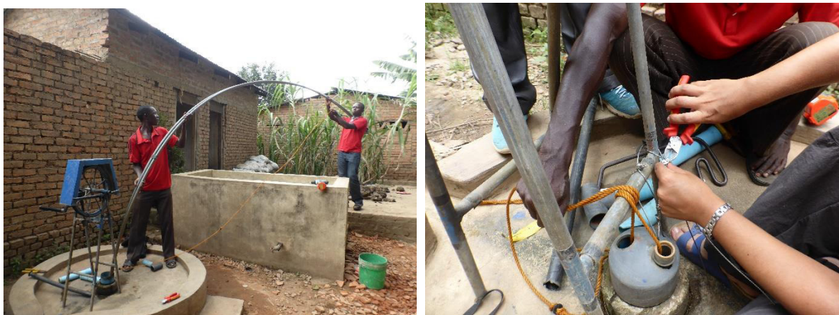
Fig. 4.3: Installation of pressure data loggers in a pumping well in the Ifakara study site (pictures: G. Gabiri).
