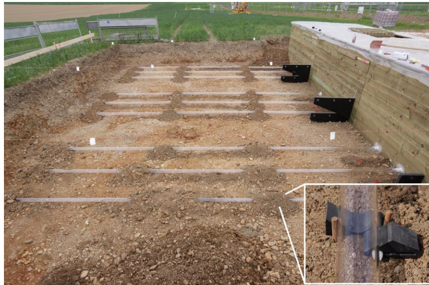
Fig. 2. 1 Installation of the minirhizotron facility in the upper part of the test site. The wood container is the accessible facility. Wedge-shaped fixture blocks shown in the right corner were used to fix the tubes during soil backfill.
