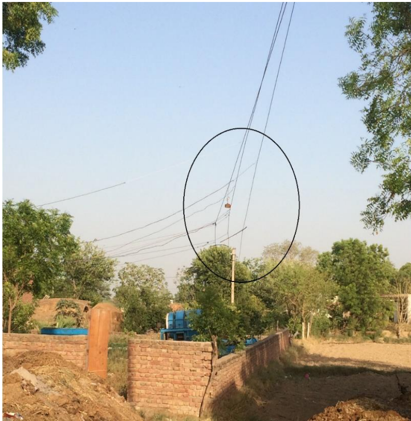
Figure 2.4: Field Observation- Electricity thefts
