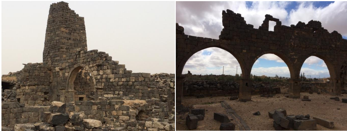
Fig. 2.5: Part of Umm el-Jimal ruins totally built of basalt as the entire site.
