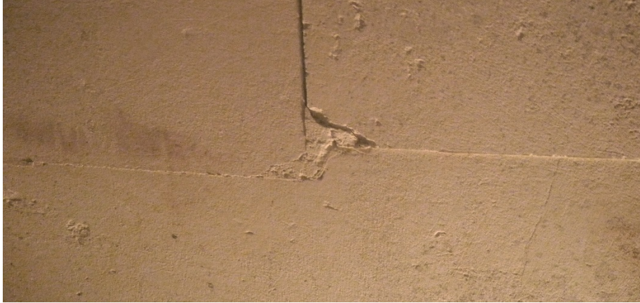
Fig. 17. Horizontal block edge with a small step, from the underground burial apartments of Khenemetneferhedjet Weret II.
