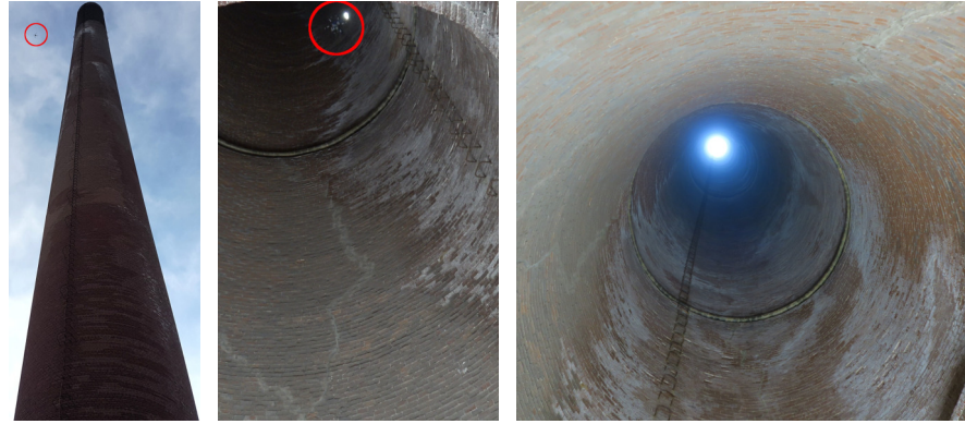
Figure 5.3: Industrial chimney inspection. Surface inspection in industrial chimneys with MAVs requires safe navigation in proximity to the surface in a small confined space. The perspective of a pilot on the bottom of a chimney makes flight maneuvers in larger heights hard to control without automation (MAV circled red). Left: Manual chimney inspection from the outside in larger distance from the wall is not suitable for 3D surface reconstruction. Center: Autonomous flight close to the walls. Right: Manual operation in larger heights inside the chimney is prohibitive, especially in daylight conditions.
