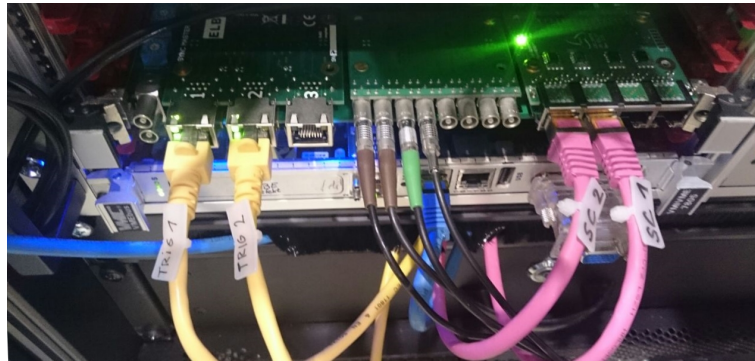
Figure 9.2.: Close-up view of the ELB-VME-VFB board, with the Sync Master on the left, an eight-fold NIM output in the middle, and a four-channel Slowcontrol Extension (see section 6.5) on the right. One of the trigger (yellow) and slowcontrol (magenta) cables connect to each of the two Backplanes.
