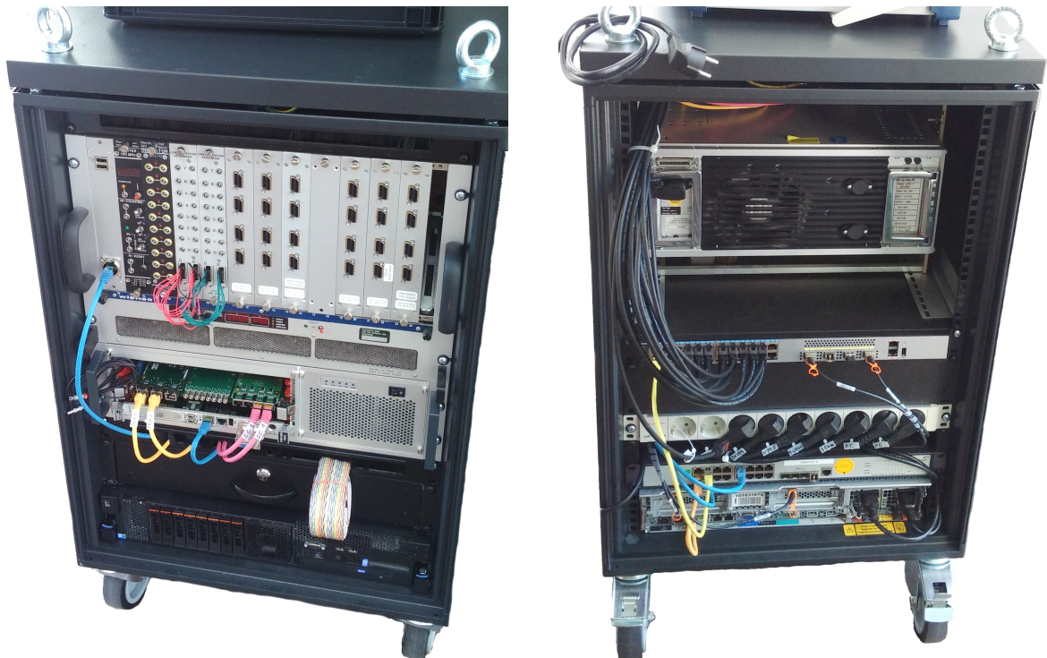
(a) Front, showing six CB-SADCs in the NIM crate, the VME crate, a drawer, and the cbsadcserver . (b) Back, additionally showing the two Ethernet switches and the power distribution.
